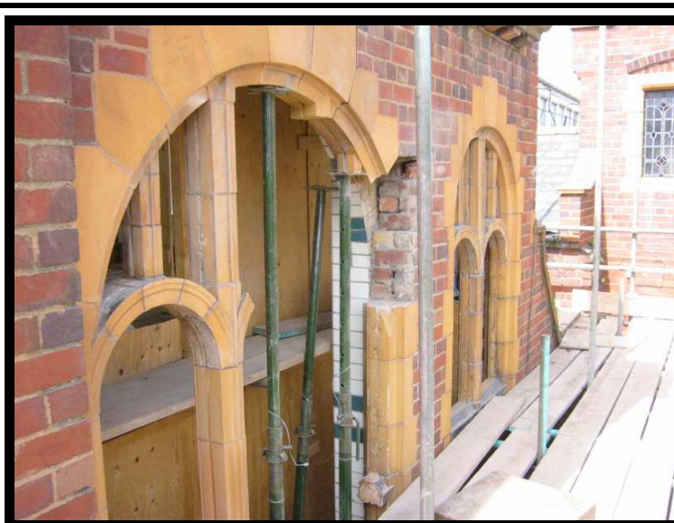
The above photograph shows the rebuilding of the terracotta windows in Pool 2. New terracotta blocks have been made to replace any that have crumbled.
